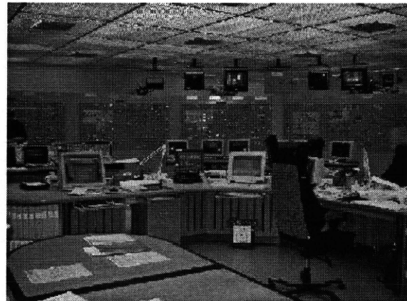
Figure 1: A view of the Main Control-Room
